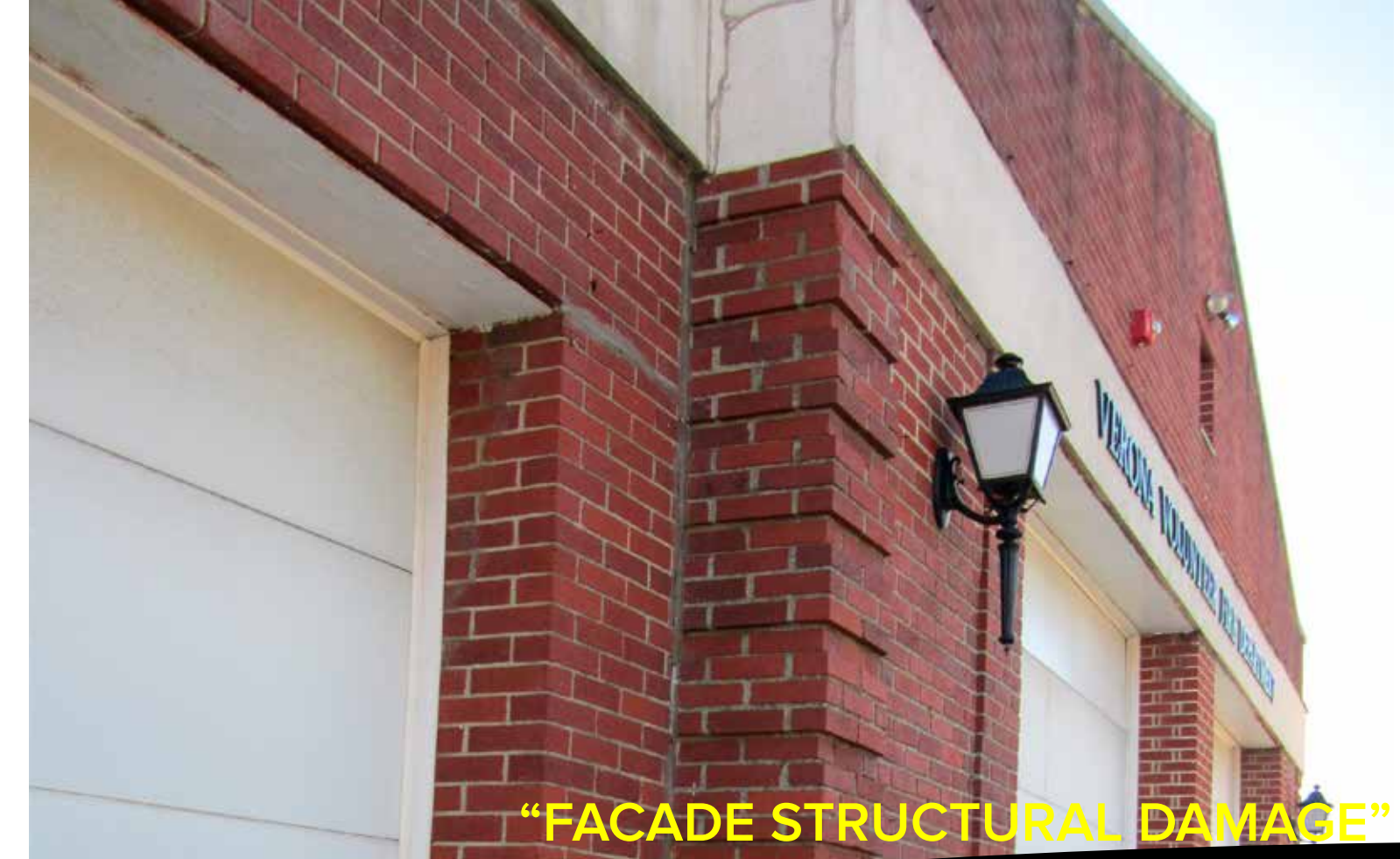
"FACADE STRUCTURAL DAMAGE"
