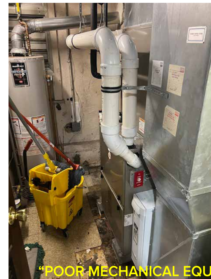
"INADEQUATE WORK AREAS"
